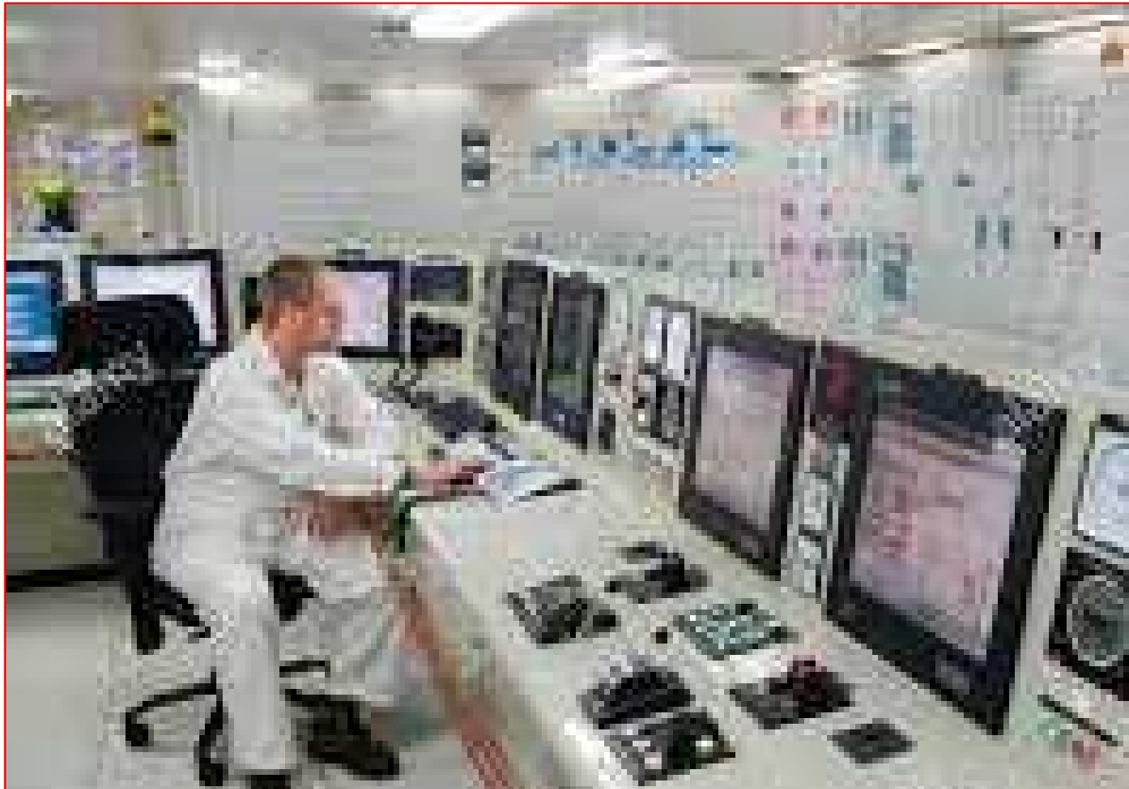
AUTOMATED ENGINE CONTROL ROOM ENGINE ROOMS , MACHINERY NOT MANNED
